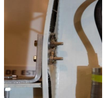
Figure 11 - Mat torn and punching shear of washer.
